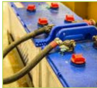
Lead Acid Batteries
