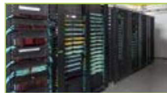
Servers and Server Cabinets
