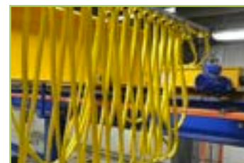
Overhead Crane Cables
